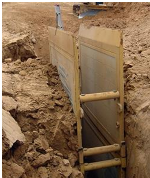
This trench box saved an employee's life when the dirt walls around him collapsed. Photo credit: Underground Safety Equipment/NAXSA
